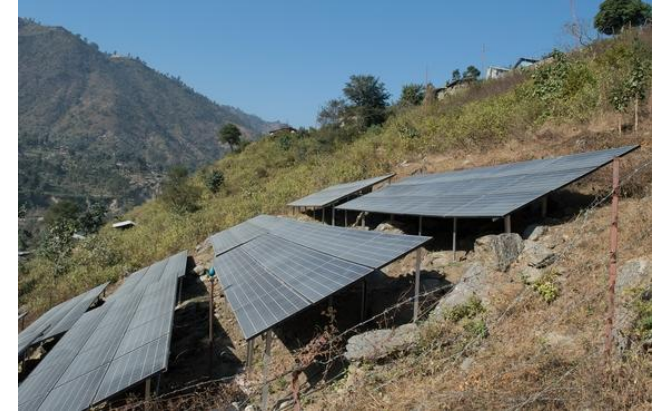
(Mini-red solar fotovoltaica en Okhaldunga, Nepal © Gham Power)
